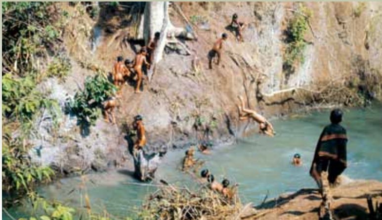
Some 41st CA Teams dammed creeks to create a swimming hole for children. Although simple, they helped to keep the children clean, and earned the CA Teams tremendous goodwill among the population.
