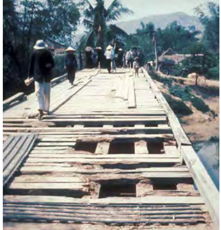
During the Tet Offensive, the security situation throughout South Vietnam deteriorated. Here is one of Team 14's bridge projects that was damaged by the VC.
