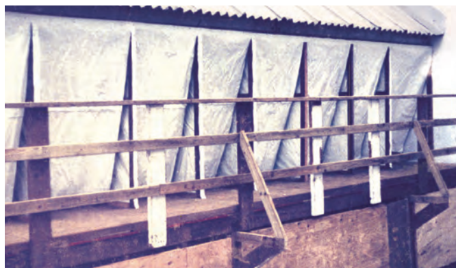
After engineers constructed toilets, MAJ Cheek had partitions and privacy screens installed.
