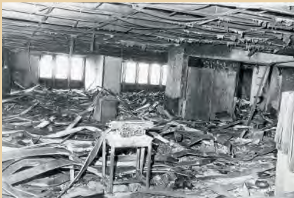
The aftermath of the 6 November 1985 M-19 seizure of the Palace of Justice in Bogotá. In a heavy-handed intervention, the Army cleared the building of insurgents, at a loss of over a hundred people; government workers, soldiers, guerrillas, and eleven Supreme Court justices.
